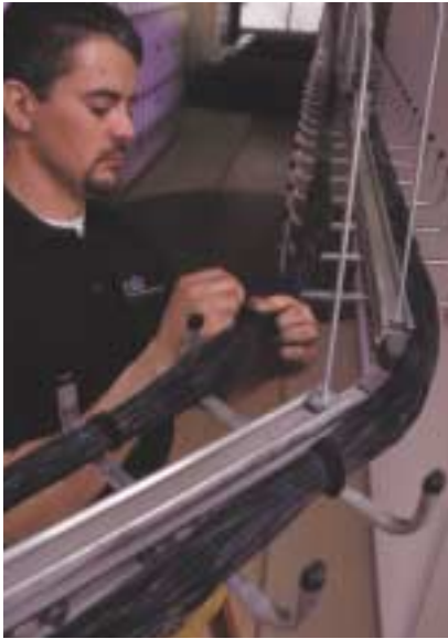
Juniper utilized the open ceiling design with runs in overhead cable raceways. To support its 100BASE-T Ethernet network, KRONE fiber-optic backbone links all four floors of the building.
