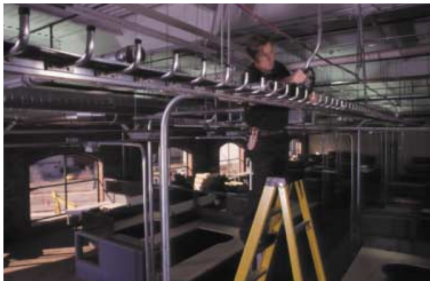
On each floor, the TrueNet C5eT cabling is channeled through a central spline cable tray, wholly visible through the building’s open-ceiling design. To accommodate Juniper’s signature color scheme, the cabling was ordered in a non-standard custom color.
